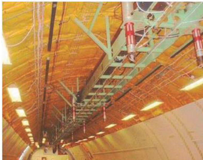
Figure 6.3. ULD fire suppression system, showing penetrators at each ULD position
